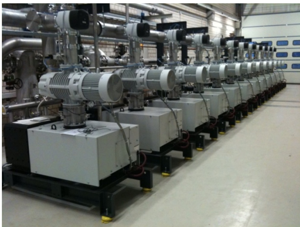
Helium compressors installed
