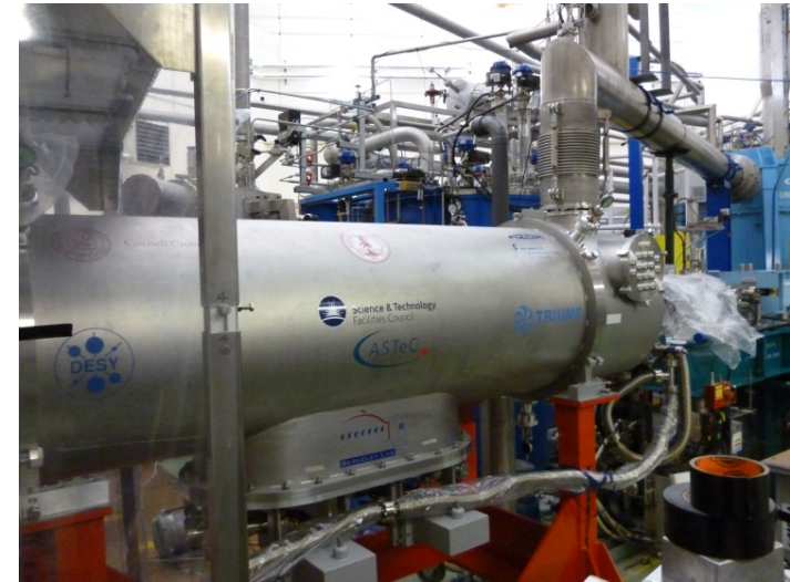
Cryomodule installed on ALICE
