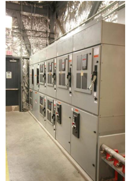
Motor Control Center
