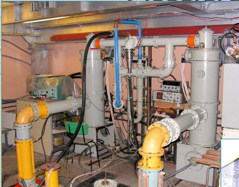
Two generators with feeders
