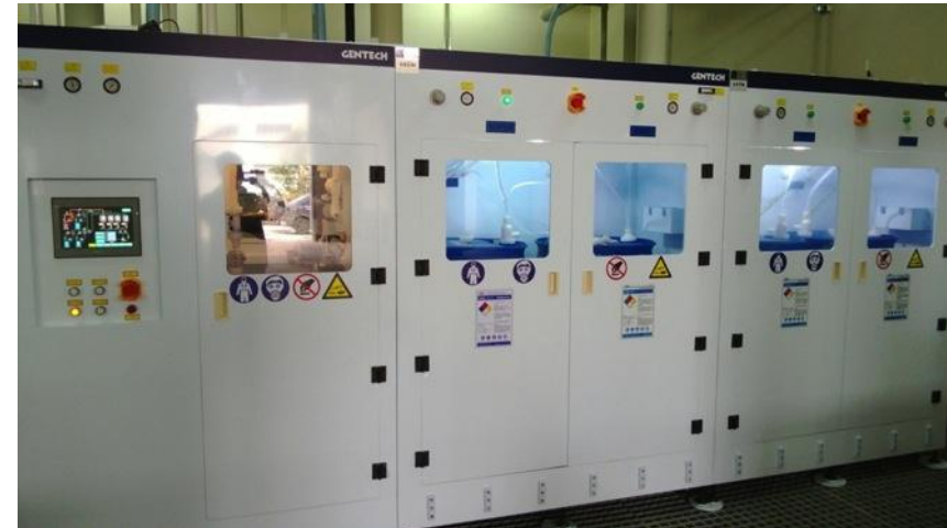
BCP acids mixing system
