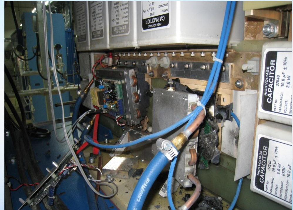
M02 A phase IGBT blasting
