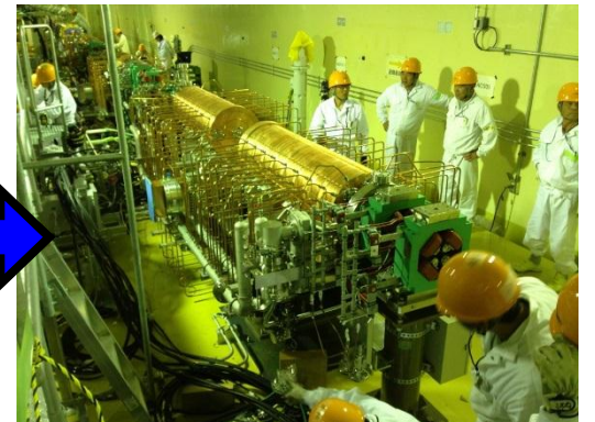
Set on the beam line
