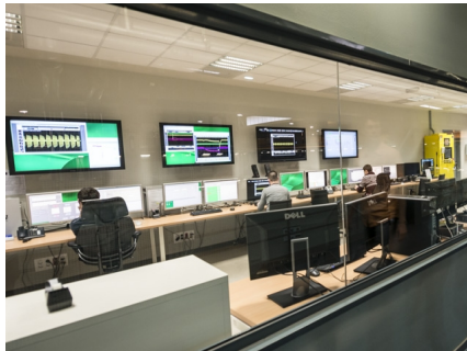
The ALBA control room
