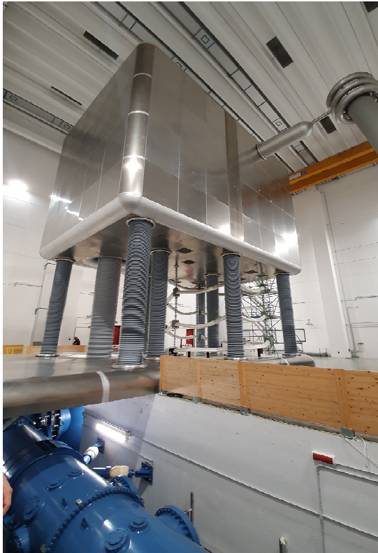
High voltage platform – DC beam
